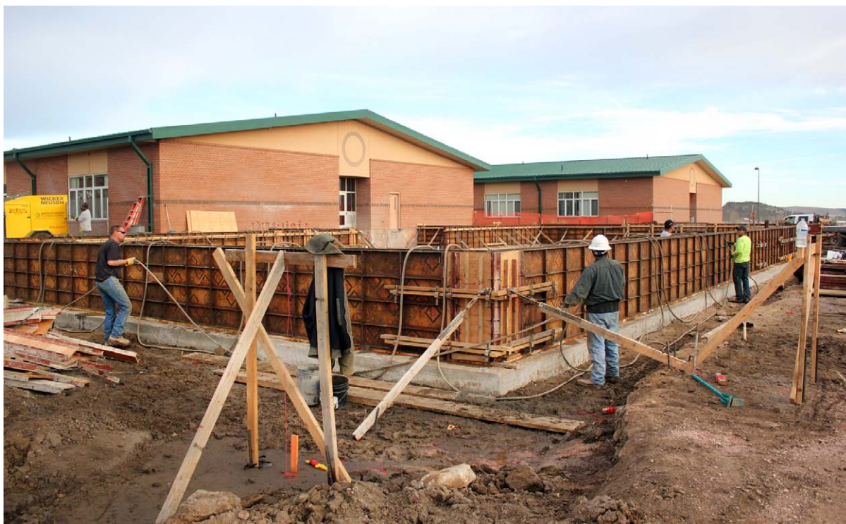
Van Ewing Construction crew is hard at work preparing the foundation for the Newcastle Elementary School addition last week.
