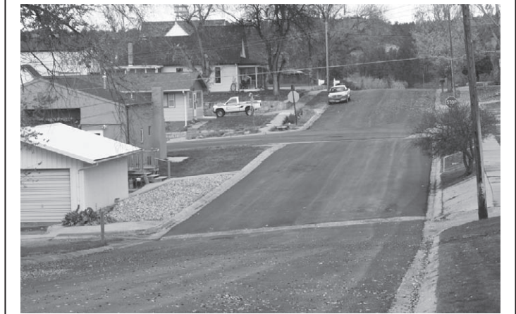
Wentworth Street and Sumner Avenue are freshly paved after months of road work. (Stephanie Bonnar/NLJ)
