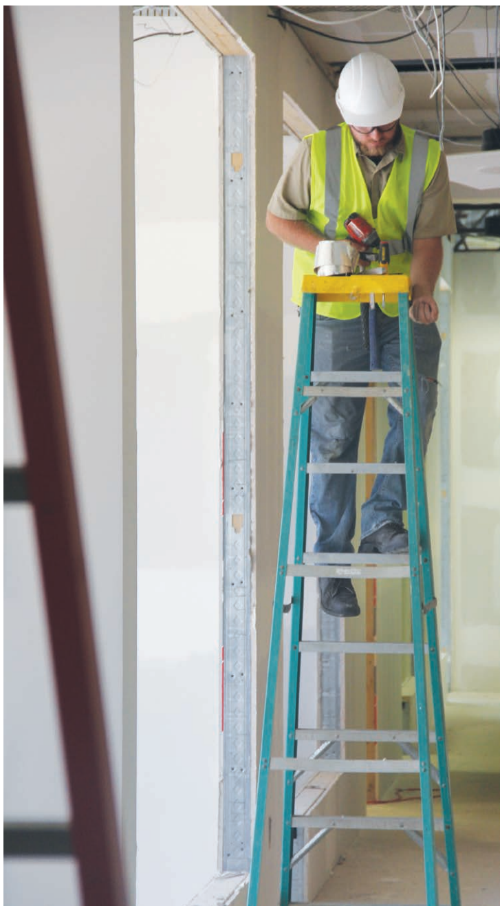
Workers with RCS Construction out of Rapid City continue with phase 1 of the First State Bank remodel project. The project will be completed over 3 different phases and will upgrade the building for better employee function and customer satisfaction. (Photo by Alexis Barker/NLJ)
