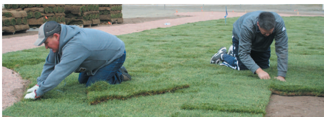
Roy Domina and Chad Ostenson wrestle rolls of sod into place at the Newcastle Baseball Complex in October. Babe Ruth players and parents lent their efforts to laying new sod on the field in the fall, and they hope to raise enough money to install new lights before the season begins this summer. (Bob Bonnar/NLJ)
