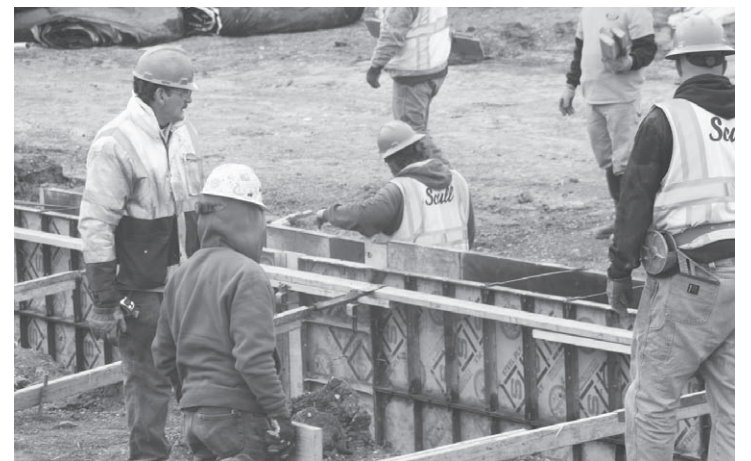
Workers brave cold temps to lay out forms for the pouring of a new foundation at WCHS. (Pam Penfield/NLJ)
