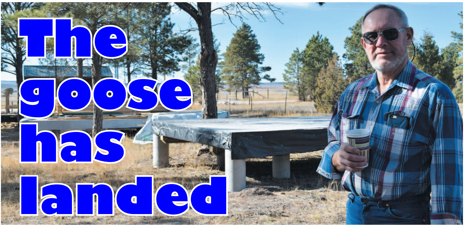
Dave Gose stands near five rental cabins currently under construction on the property of his Goose Landing archery range. The Upton native, who divides his time between here and Alaska, plans the multifaceted facility as a regional draw that will provide camping and other recreational opportunities in addition to indoor and outdoor archery. (Todd Bennington/NLJ)
