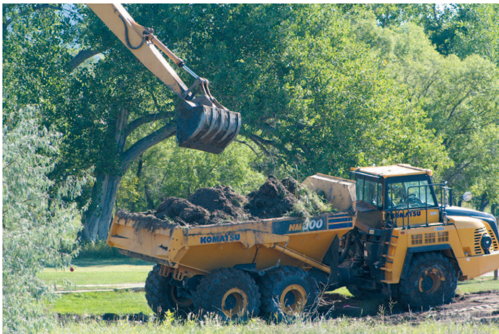
Crews are spending this week removing the top layer of soil and vegetation from the lowland area so it can be used as topsoil on the area surrounding the pond. (Alexis Shultz/NLJ)
