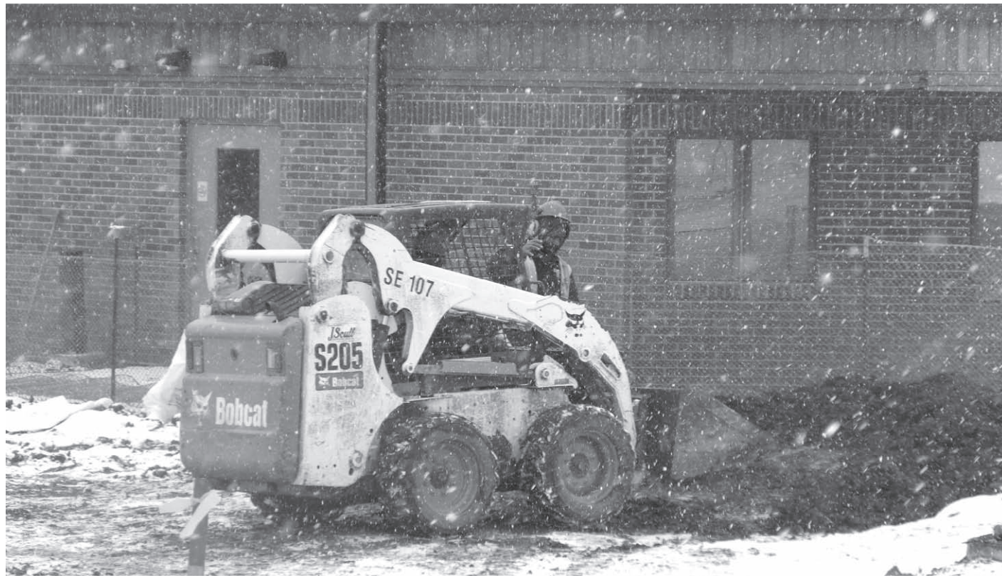
Hospital construction is in full swing, even on the snowy morning of January 14th. Despite the week of winter weather, crews have been making progress on building renovations. The hospital is still accessible via the alternate entrance on Boyd Avenue. (Jessica Yarnes/NLJ)
