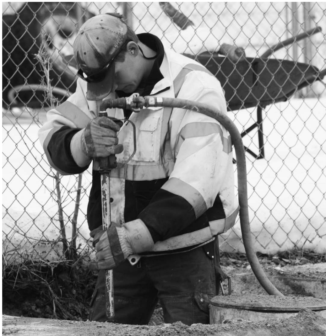
Scott Lindstrom uses a jet of water to loosen the soil around a broken water line in Frontier Addition on Monday. A leak at the curb stop at 104 Frontier Street caused a decent amount of ice to build up on the street over the weekend. City Engineer Mike Moore told the News Letter Journal that the leak began some time last Thursday evening, and city crews put out a ground-heater to thaw the ground over the weekend to begin working on the leak on Monday. Moore reported on Tuesday that the leak has been fixed, and that crews discovered it was caused by the water line pulling away from the curb stop. (Alexis Barker/NLJ)
